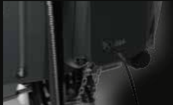
Battery charger on board
